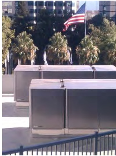
Figure 1: 10 units of 120 kw fuel cells are installed on the top floor of Adobe headquarters in San Jose, photo Edelman
